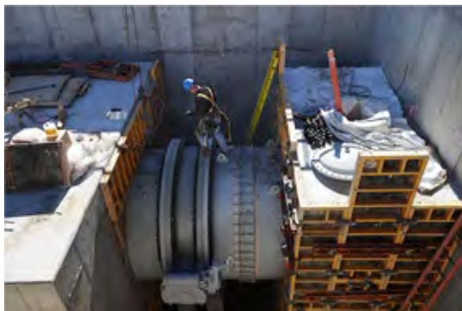
MWWST Valve Vault and Pipeline
